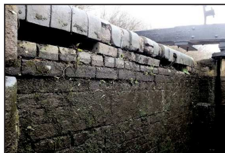
The Gate recess of lock 3 months before the gate failed
