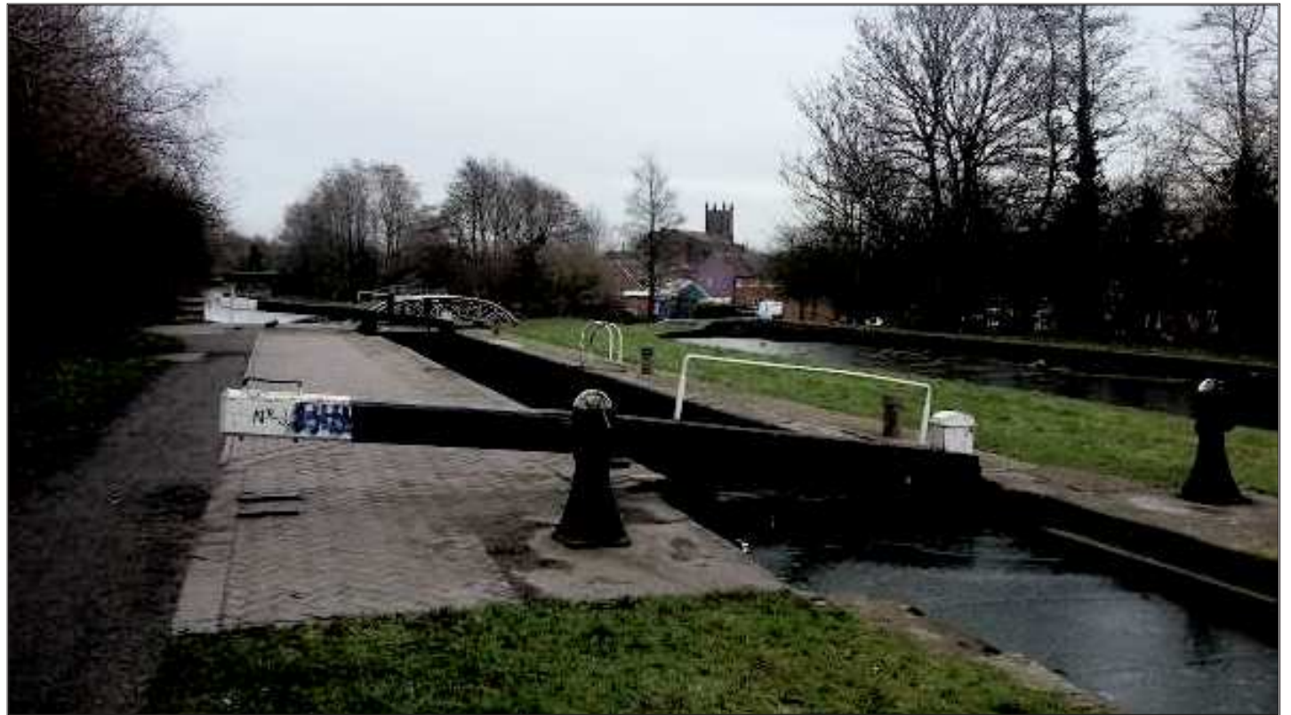
The failed lock at Tipton, pictured in February before it finally became too dangerous to ignore.
